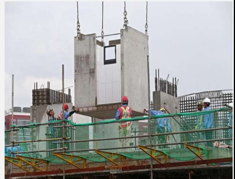
Prefabricated bathroom units are assembled with finishes in a factory before it is transported to a construction site for installation.
